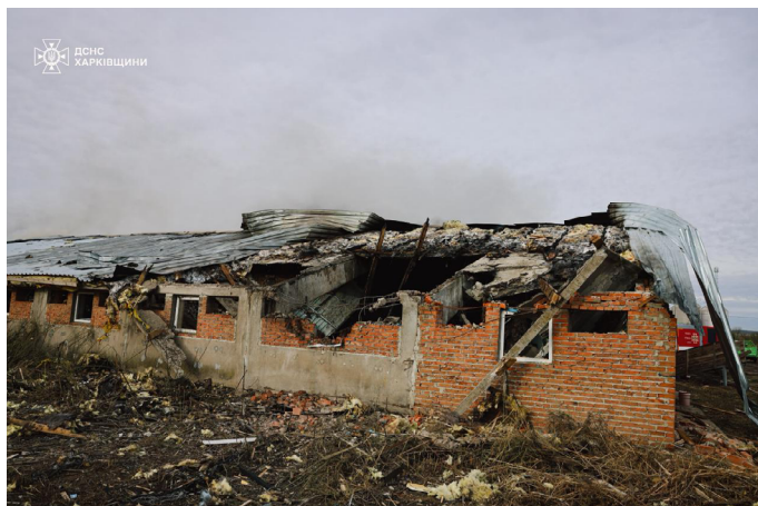
Agricultural facility destroyed in a massive drone attack by the russian army in the Novovodolazka hromada Photo: State Emergency Service of Ukraine
