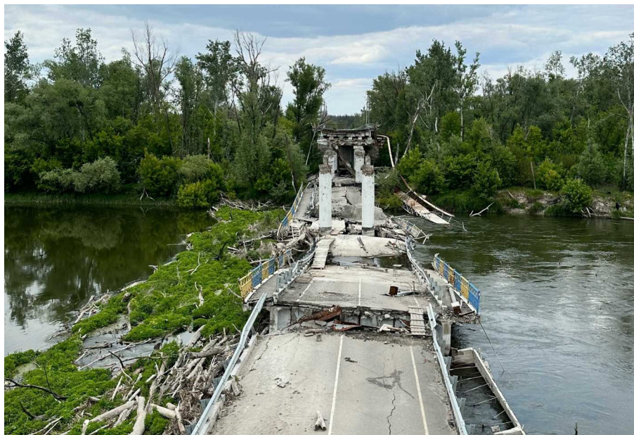
Destroyed bridge in Bohorodychne village, Donetsk Oblast
