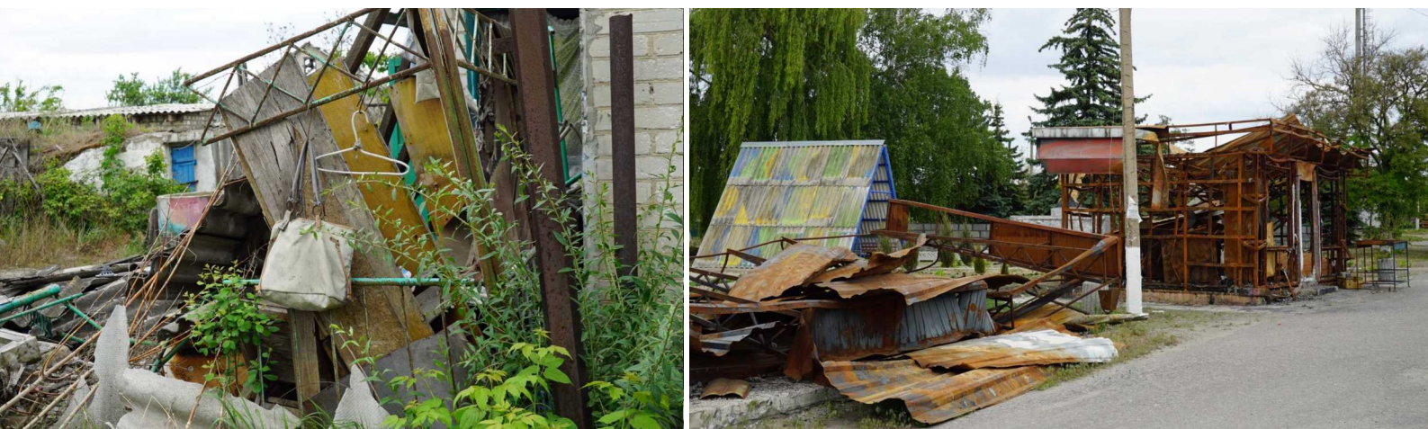
Destroyed houses in Yarova village, Donetsk Oblast
